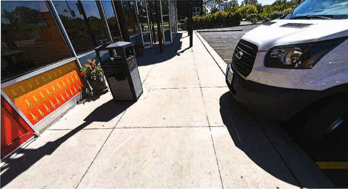
Overhang of parking into the proposed sidewalk
